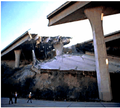
(Source of Photo: FEMA)
