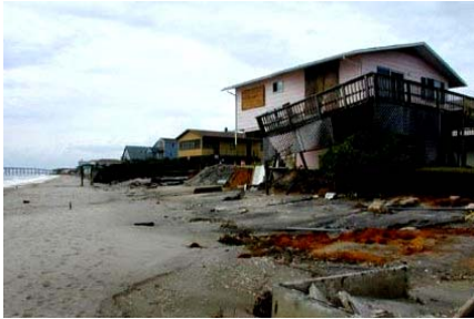
(Source of Photo: FEMA)
