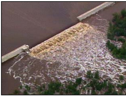
Flooding across the spill way at Buckhorn Dam on September 17, 1999
