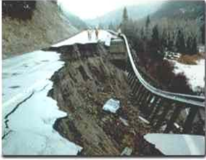
(Road failure caused by a landslide. Source of Photo: NOAA.)
